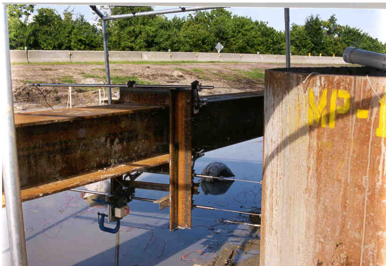
LVDT's and string potentiometer mounted to independent reference beam for lateral Statnamic test.
