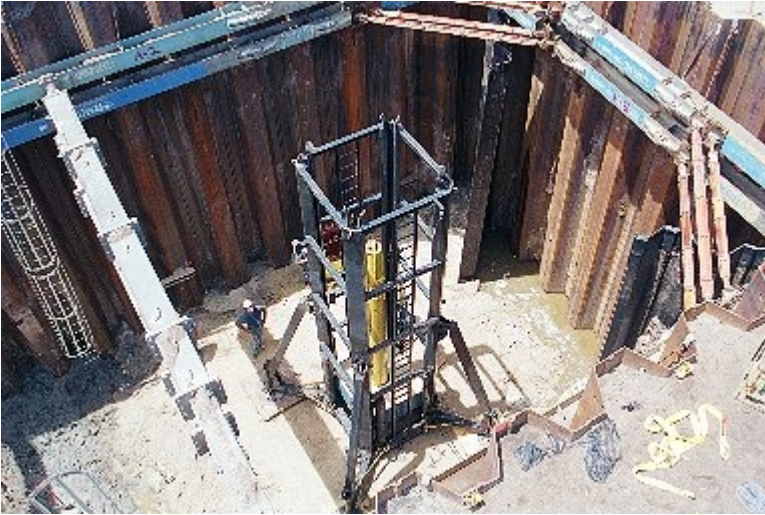
Catch mechanism STATNAMIC load test on an 18" square concrete pile within a coffer dam. US Army Corps of Engineers.
