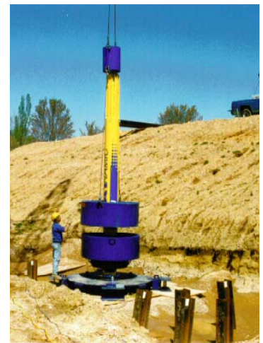
1997 — AFT's first STATNAMIC load test. Testing H-Pile for a Bridge project in Poplar Bluff, Missouri, MoDOT using a gravel catch system.
